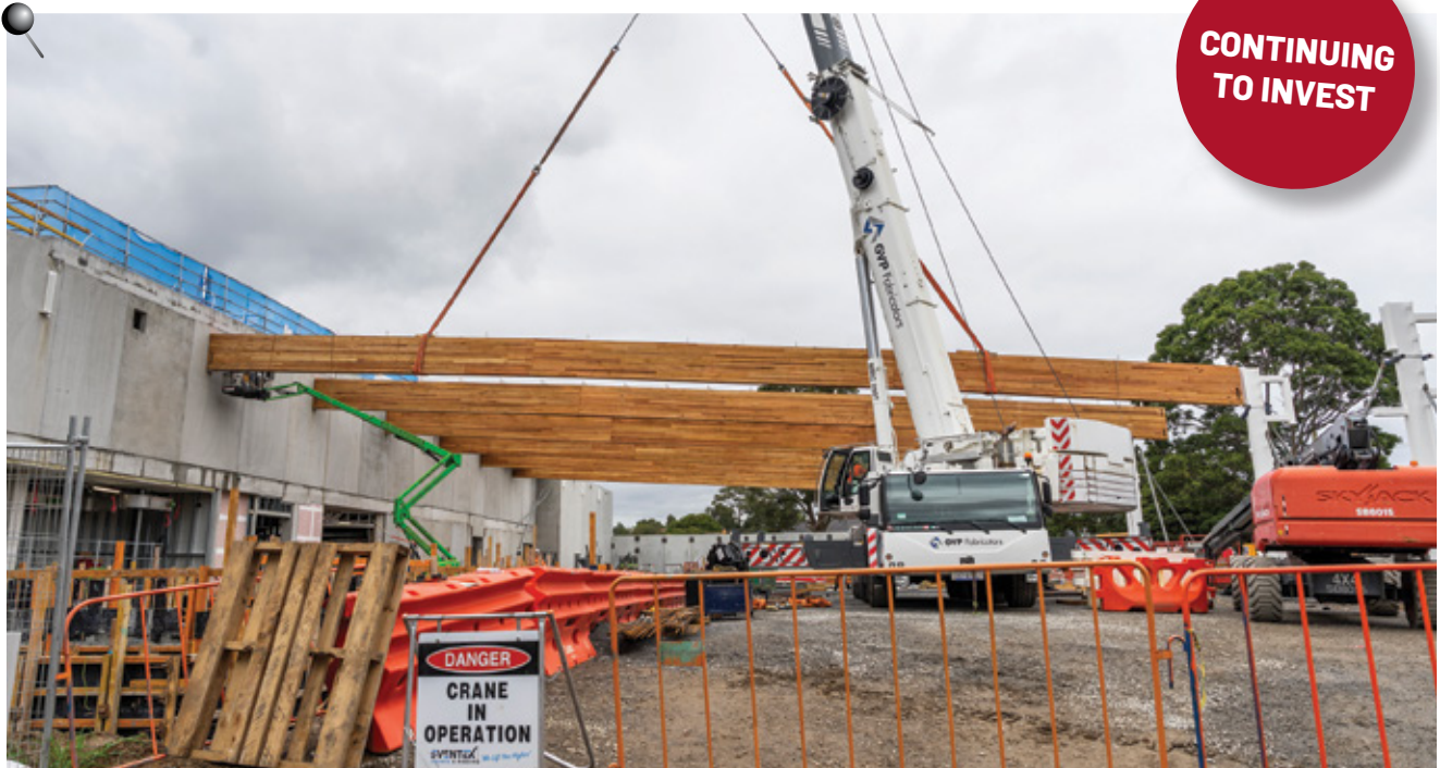
A crane lowers a massive timber beam into place at Oasis Aquatics and Wellbeing.
